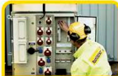
Power and heating
