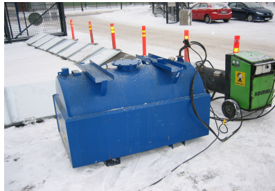
Power and Heating
